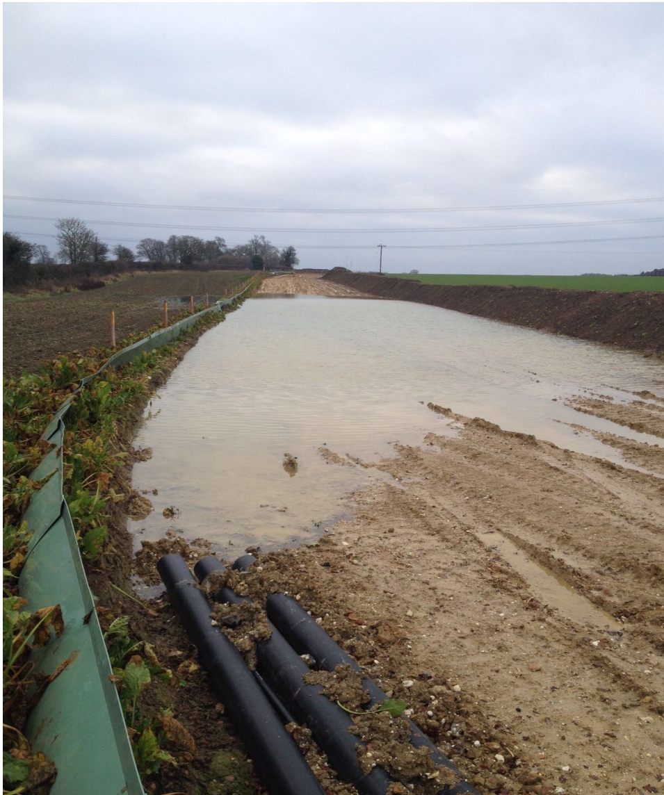
Figure 3 Land drains will have to be cut to lay cables, leading to flooding in areas in and around the cable corridor
