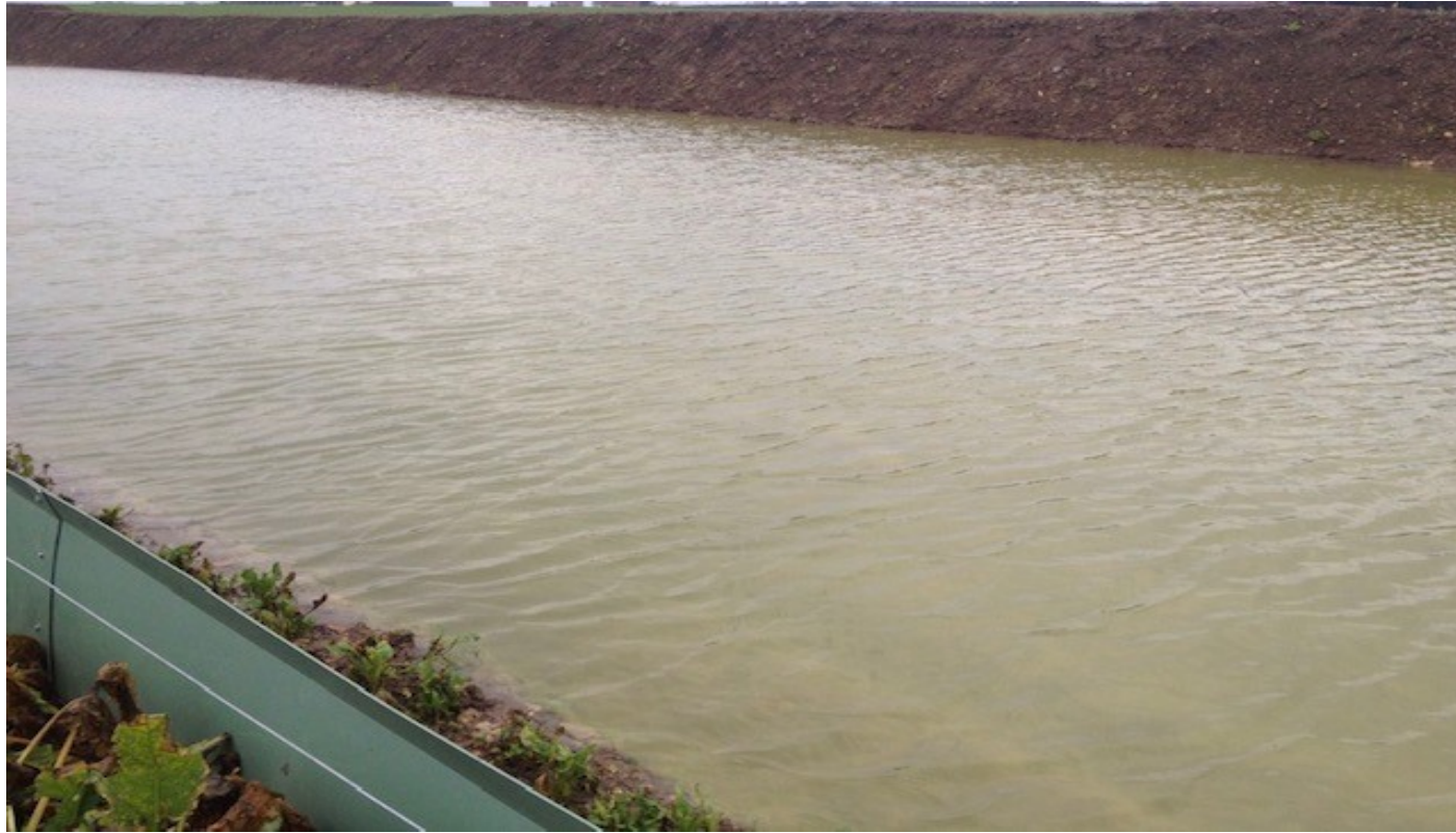
Figure 4 Dudgeon Offshore Wind Farm cable corridor – 32 land drains cut in just one field
