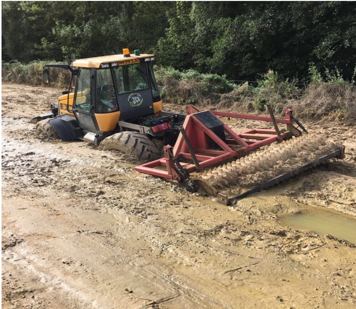
Figure 1 Soil damage in the wide cable route areas
